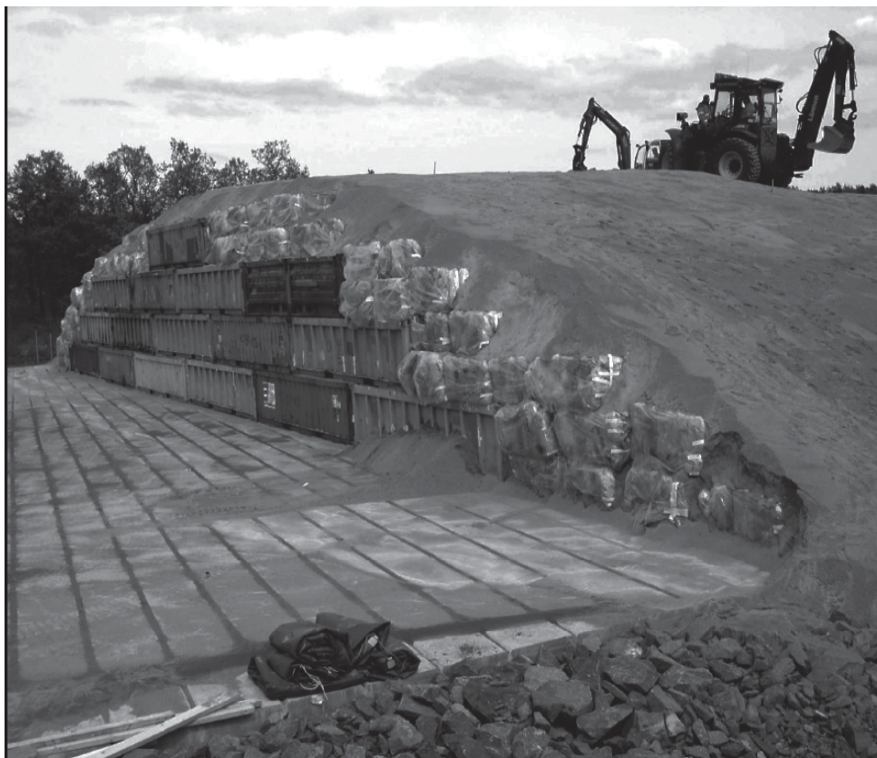
Figure A1.3: Disposal facility for VLLW at the Oskarshamn nuclear power plant (Sweden)
