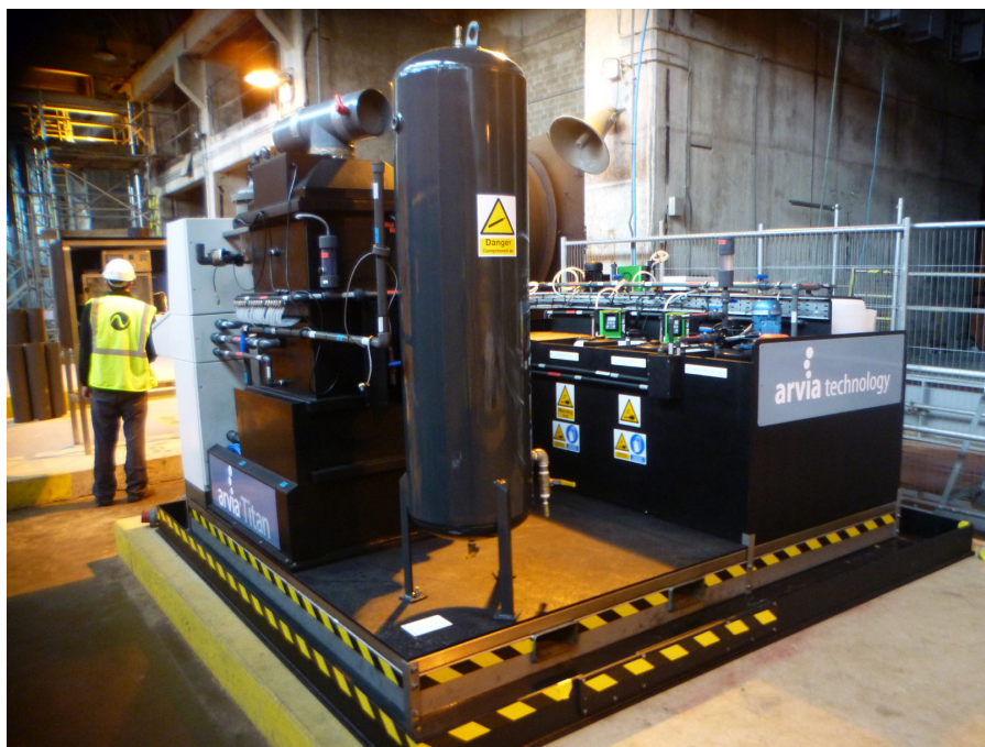
Figure 5.4: The Arvia® Titan on site at Trawsfynydd
