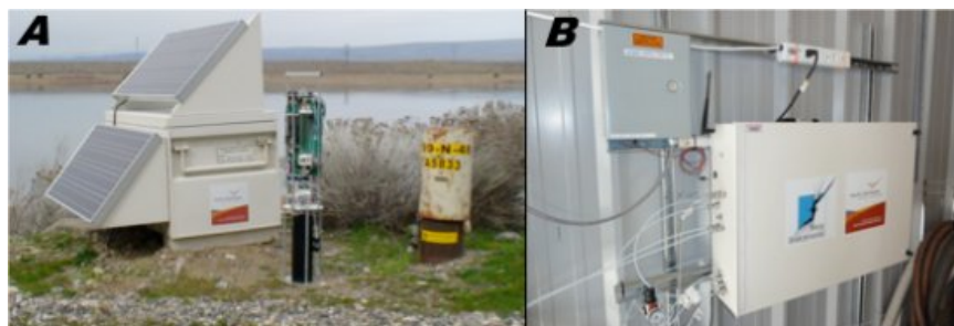
Figure 6.26: Hanford's prototype ^{90}\text{Sr} monitor and ^{99}\text{Tc} pump and treat process monitor
