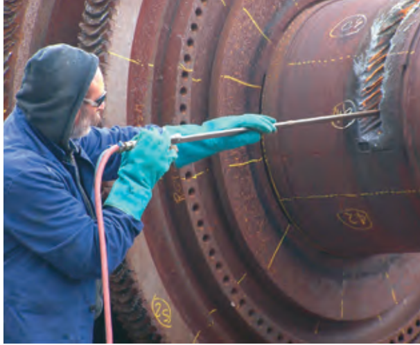
Segmenting large plant items during the dismantling of the cooling towers for residual heat removal, Caorso nuclear power plant, Italy.
