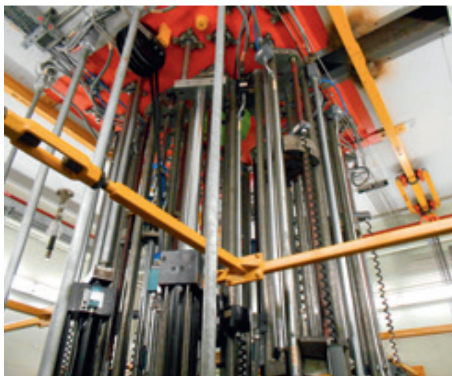
TREAT subpile room, Idaho, United States.
