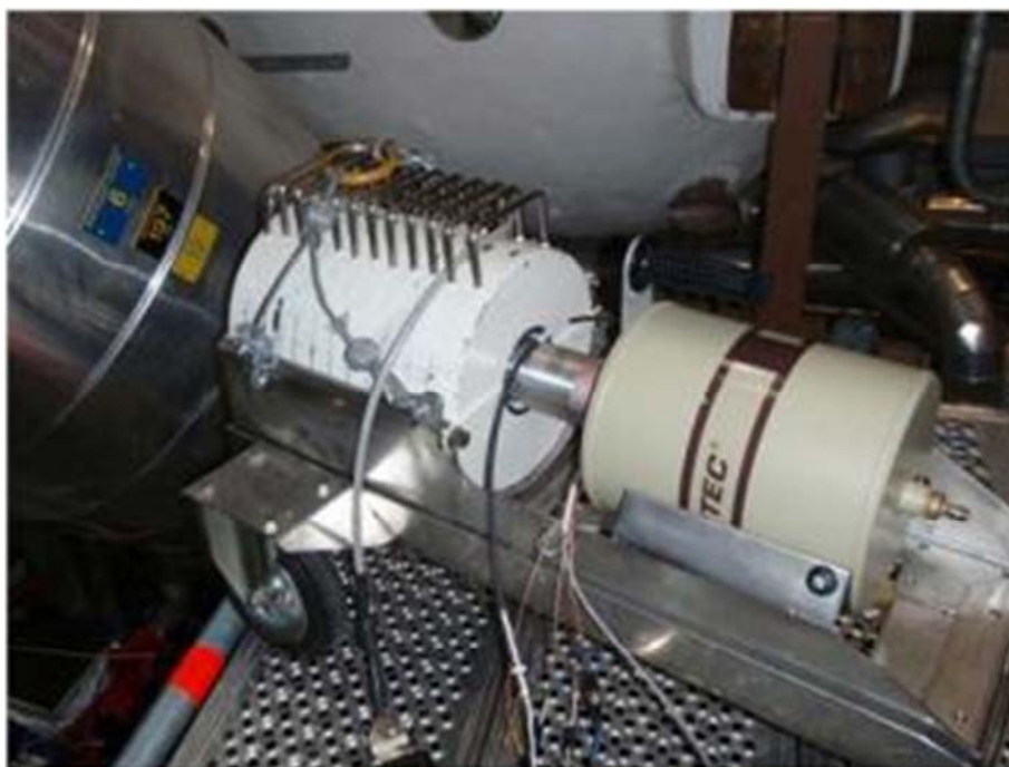
Figure 56: Portable HPGe detector with collimated shielding for a BWR MADAC based measurement campaign, here measuring on a BWR-75 steam pipe (Forsmark 3)
