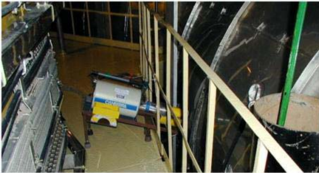
Figure 50: Steam generator measurement at Hungarian NPP Paks
