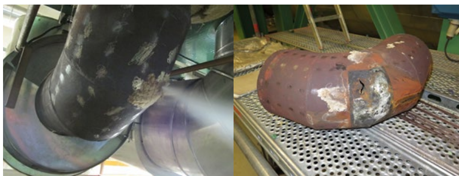
Figure 4.21. Photo of Steam Leakage and Detail of Damaged Mitered Elbow
