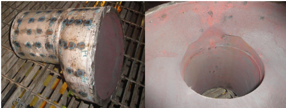
Figure 4.24. Demonstration of the FAC pipe thinning region.
