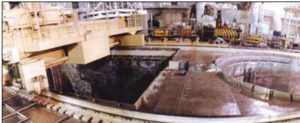
Fig. 4.3 Uncovered SF pool at NPP Temelin
