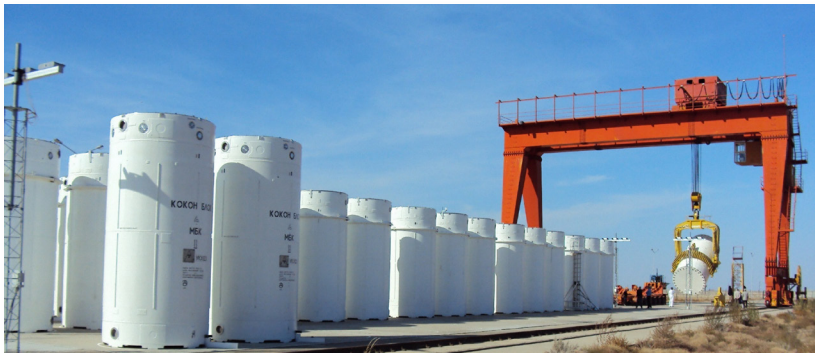
Figure 3.2. Spent fuel dry storage in casks stored outdoors in the United States
