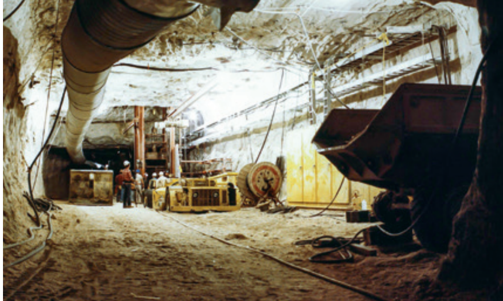
View of main drift looking north towards station at 2 150 foot level. Department of Energy, United States.
