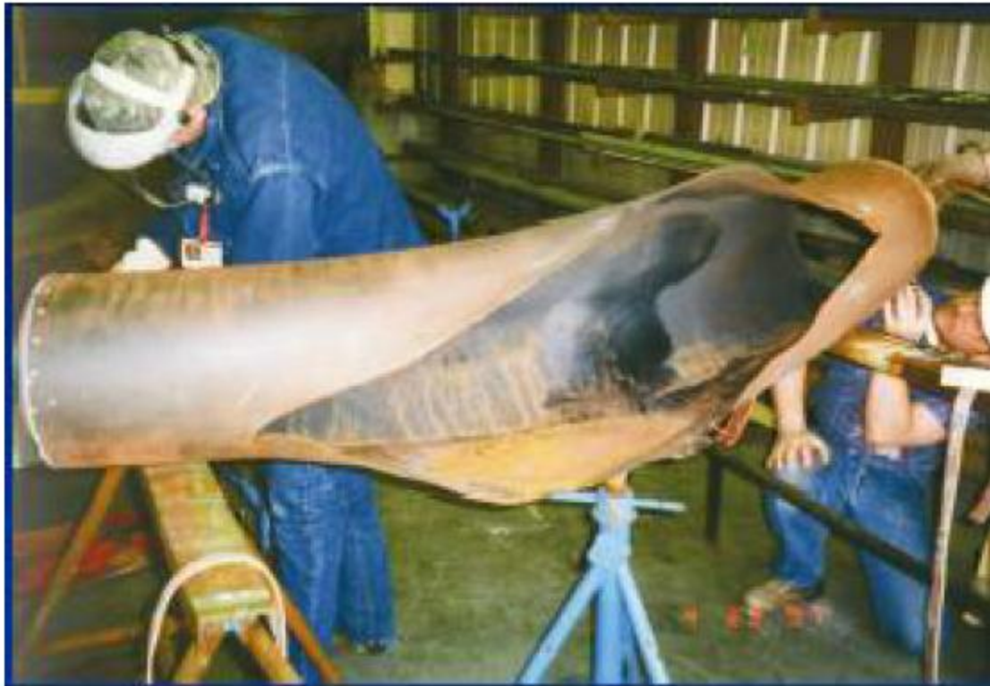
Figure A-2: Ruptured Long-Radius Elbow
