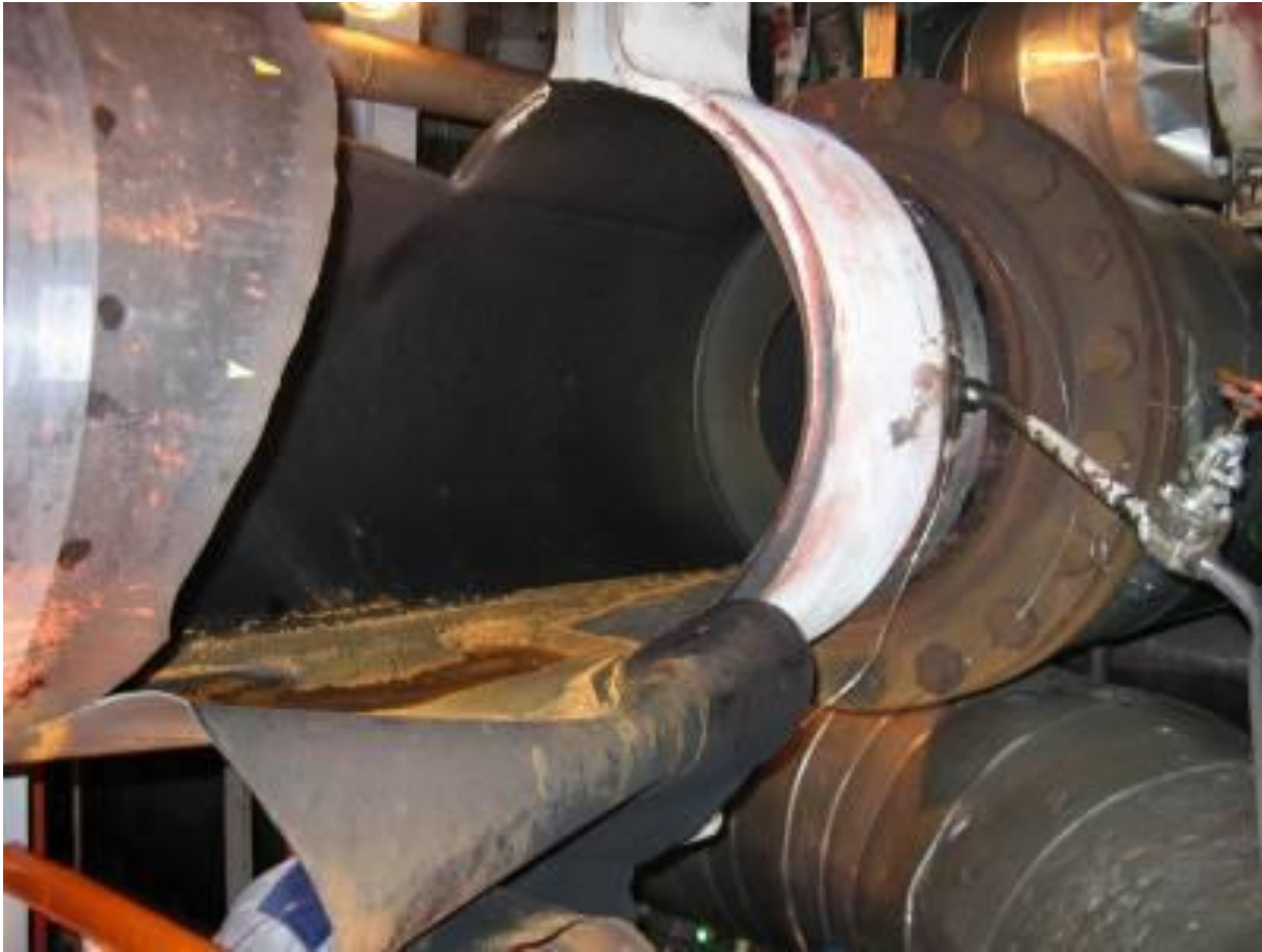
Figure A-3: Mihama-3 Condensate Pipe Failure
