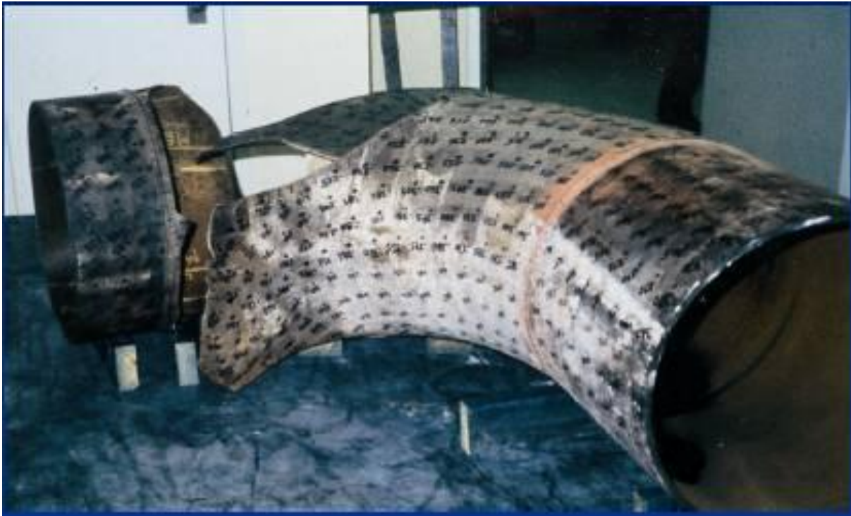
Figure A-1: Ruptured Elbow in Feedwater Line at Surry 2
