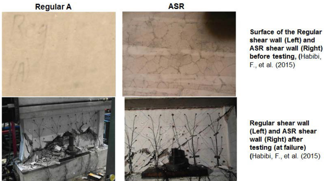
Figure 4. The first set of shear walls REG A and AAR A1 before and after testing [Habibi et al., 2015]
