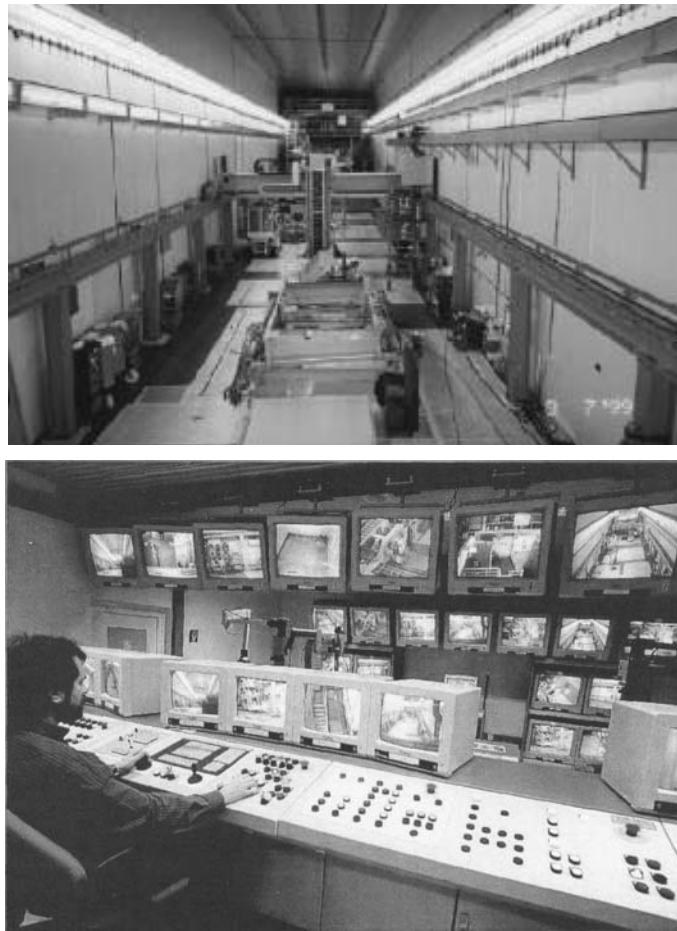
Figure 63: Crane hall above the cells, and the central control room
