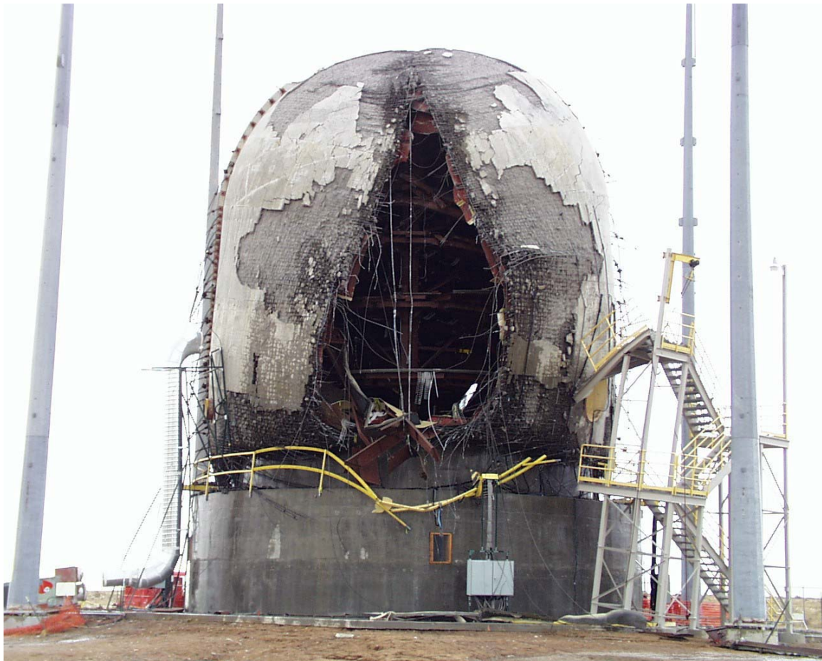
Figure 3.18 PCCV Model after the Structural Failure Mode Test
