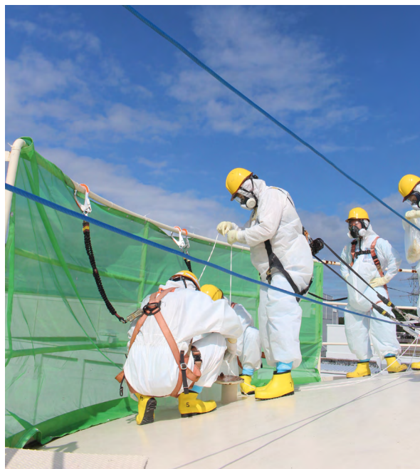
Workers maintaining a tank storing treated water on the premises of the Fukushima Daiichi Nuclear Power Plant. Source: TEPCO Holdings
