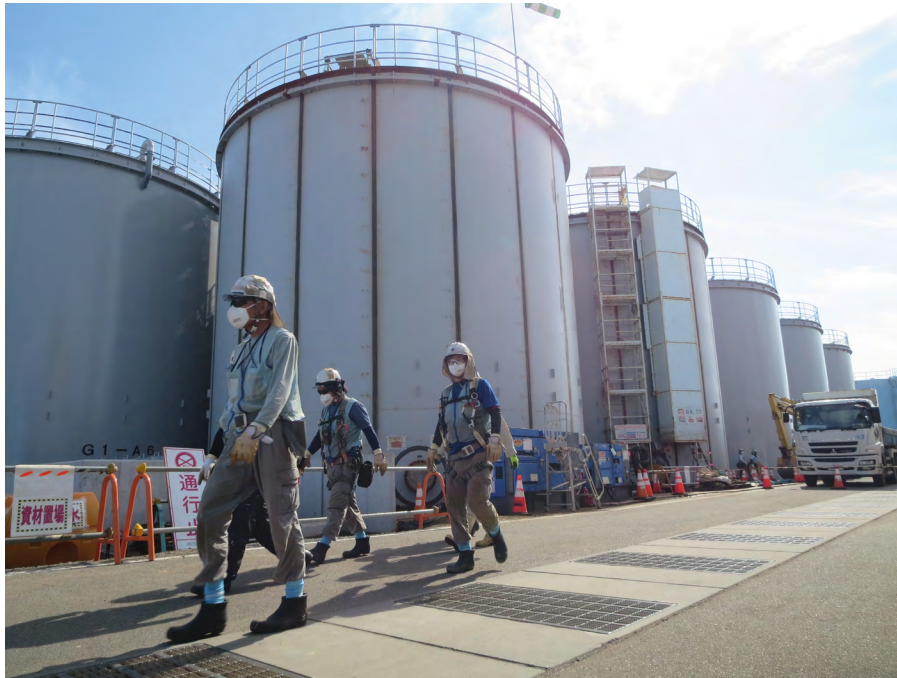
Workers performing maintenance on tanks for storing ALPS treated water installed on the premises of the Fukushima Daiichi Nuclear Power Plant. Source: TEPCO Holdings
