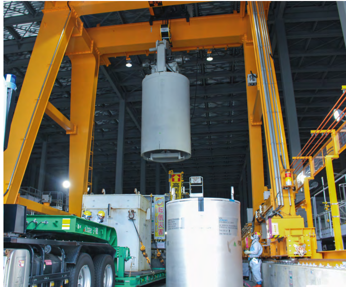
Workers handling storage containers for adsorbents used in equipment that purifies water containing radioactive substances generated on the premises of the Fukushima Daiichi Nuclear Power Plant. The used adsorbents are stored and sealed in a robust container. Source: TEPCO Holdings
