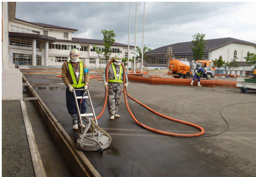
High-pressure cleaning to decontaminate the pavement surface outside the Iitate Junior High School building in Iitate Village (photo taken in July 2016). Source: Decontamination archive site, http://josen.env.go.jp/archive/detail/?IT-01-P0038
