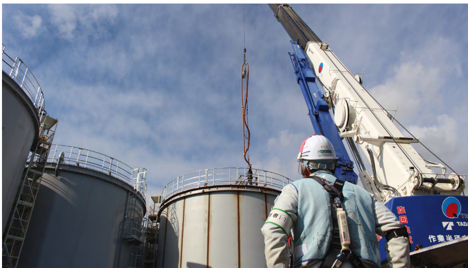
Work on a tank that stores ALPS treated water generated on the premises of the Fukushima Daiichi Nuclear Power Plant. Source: TEPCO Holdings
