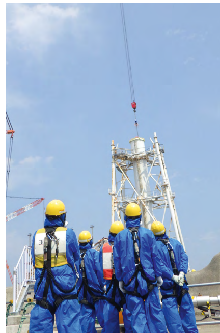
Workers dismantling the upper part of the exhaust stack of Units 1 and 2 of the Fukushima Daiichi Nuclear Power Plant. This operation was completed in May 2020. Source: TEPCO Holdings
