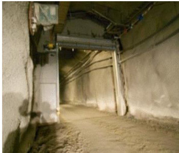
Figure 4.3: Fire door PL3003 at the Onkalo facility in Finland
