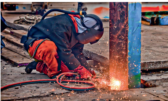
Dismantling of the Dounreay fast reactor research and development centre, United Kingdom.
