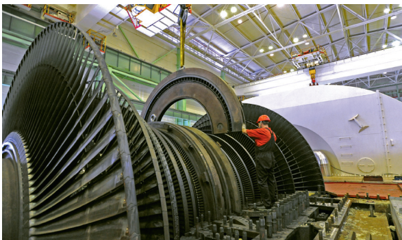
Maintenance of a low pressure section of a steam turbine at the Balakovo Nuclear Power Plant.
