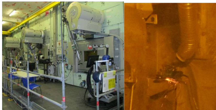
Figure B.43. Top, ELAN 2B dismantling workshop achieved using a combination of 3 telerobots paired with 3 mechanical telemanipulator MT200. Bottom, the results obtained in cutting tasks.
