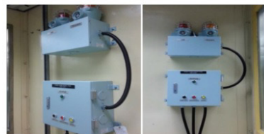
Reinforced Seismic Alarm
